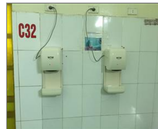
Photo of the sanitary facilities Hand drying machines.JPG
