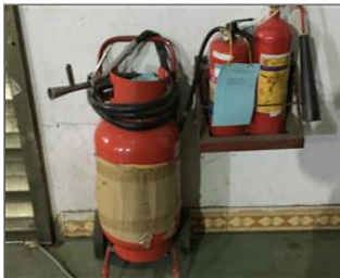
Photo of fire safety equipment Fire extinguishers.JPG
