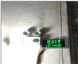
Photo of fire safety equipment Emergency and exit lights.JPG
